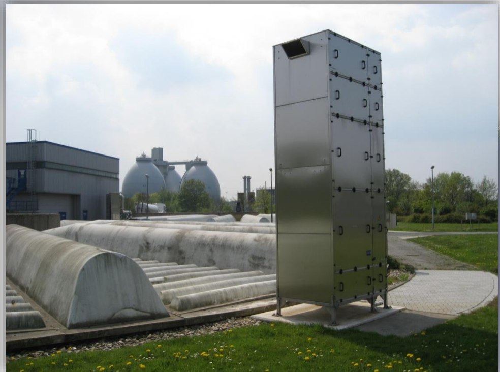
NEUTRALOX® Photoionisation at sludge holding tank
