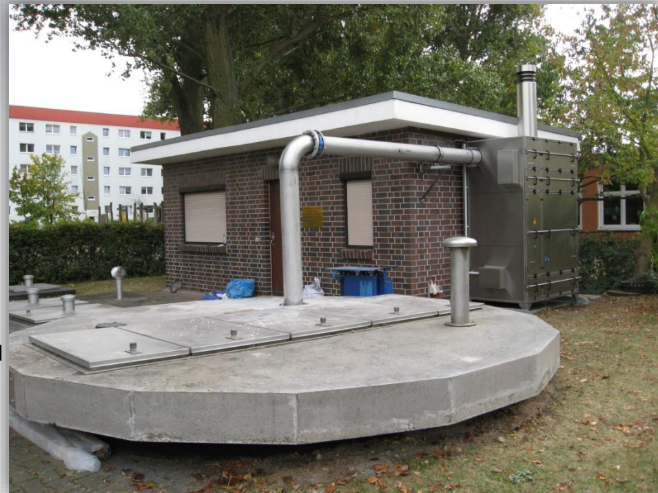
NEUTRALOX® Photoionisation at sewage pumping station
