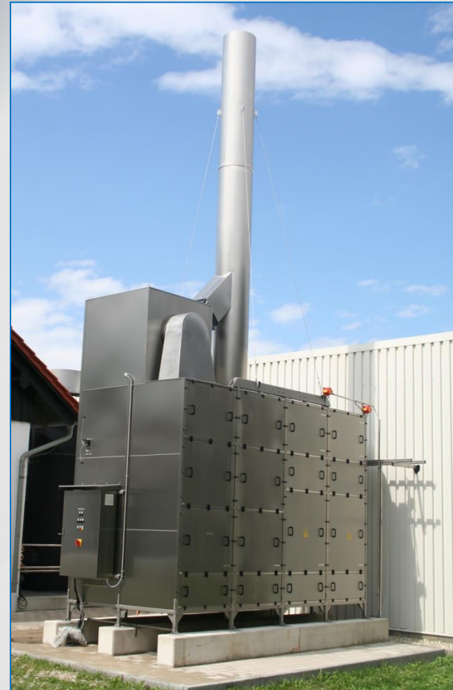
Off-gas treatment sludge dryer
